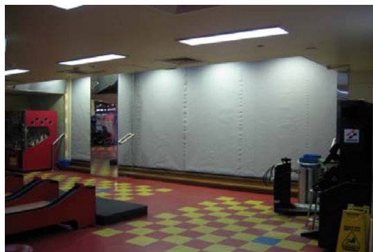
Fibershield protecting an 8.2m wide opening in a shopping centre on the Gold Coast, Queensland
